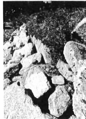
Erie Creek Dike section needing repair near highway bridge
