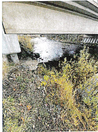
Photo 8 – Loc. 6 – Localized Scour/Erosion
